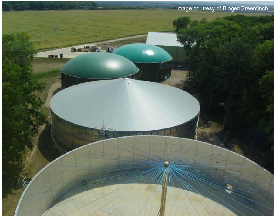
BiogenGreenfinch Digesters at Twinwoods, North Bedfordshire
